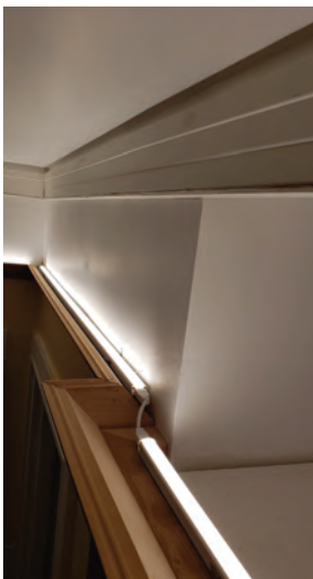
This LED strip is mounted into a channel in the crown molding and fitted with a diffuser. It provides lighting to the ceiling and the upper walls. (Photo courtesy of Eunice Noell-Waggoner)
